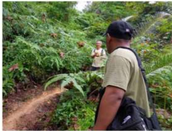
[L] Building of the Unity Trail which is the second trail sponsored by PPB Group.
